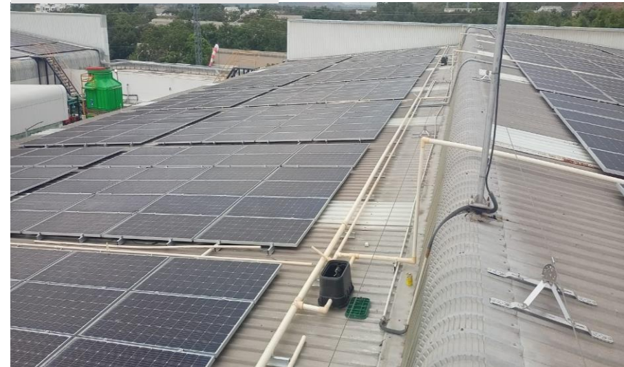
SBD1 Roof Top Solar
