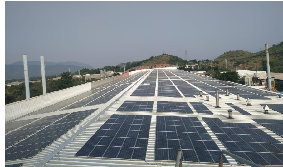
ARBD1 Roof Top Solar
